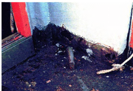
Photograph 1 Corroded accommodation house side structure
