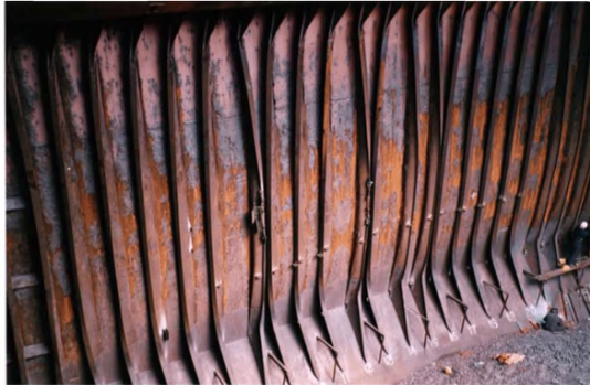
Photograph 1 Collapsed side shell frames (See Example 4)
