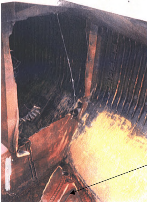
Photograph 1 Collapsed and detached transverse bulkhead
