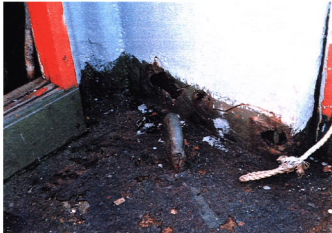
Photograph 1 Corroded accommodation house side structure
