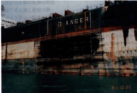
Photograph 2 Missing side shell structure (See Examples 4 and 5)
